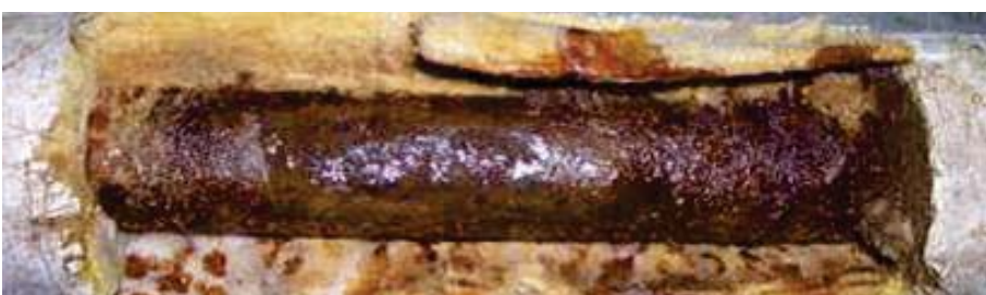
Figure 1: Corrosion under insulation
